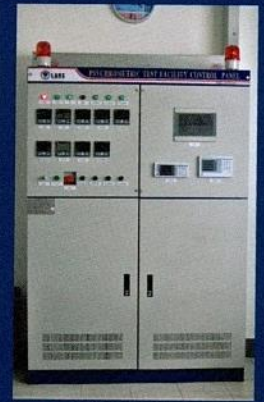
MSAT control room
